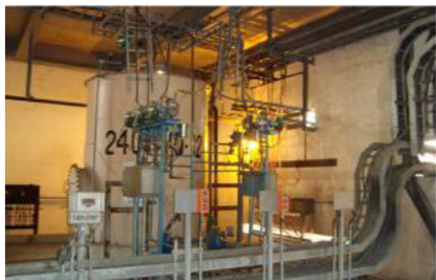
Figure 3: Dosing system with centrifugal pumps
