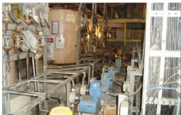
Figure 1: Dosing system with diaphragm pumps
